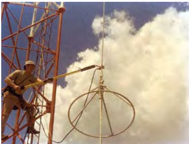
The author performing maintenance on an energized tower, LORSTA Upolo Point (Hawaii)
