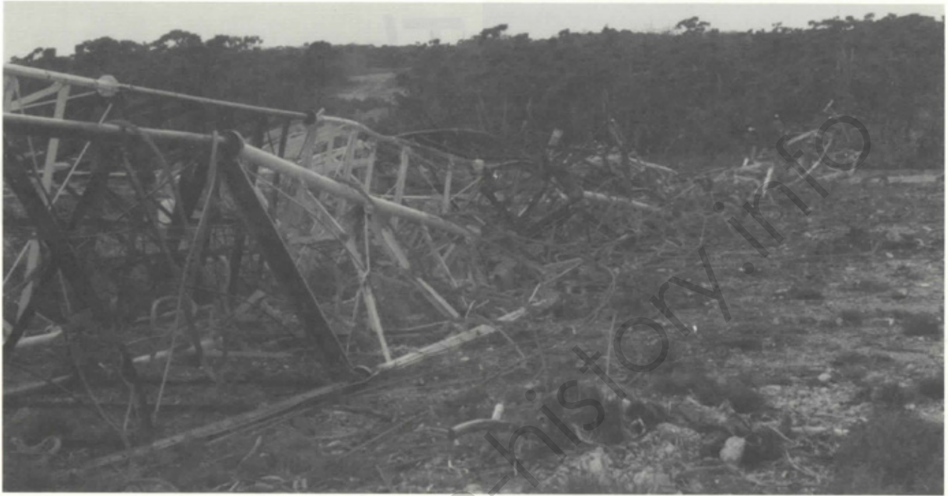
The collapsed tower lies in a heap on the ground.
