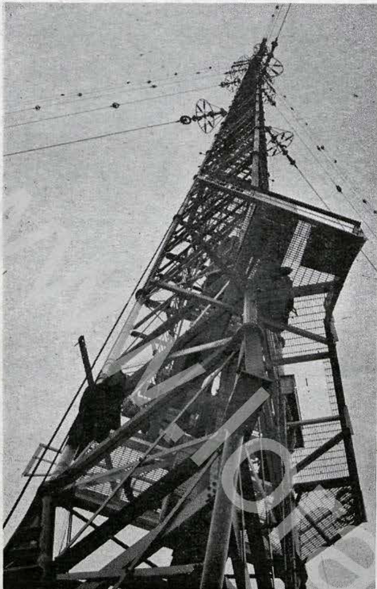
Midway in the photo is the 2-man elevator that will facilitate any future repairs. The cone-shaped corona rings prevent buildup of any charges of static electricity.
